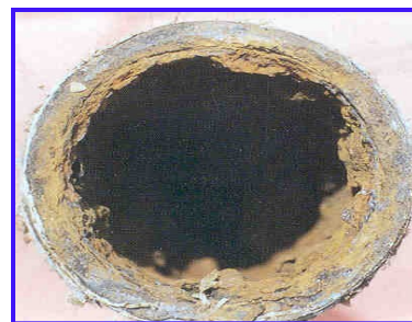
Fig.1 Heavy tuberculation and thinning of wall of FBTR
